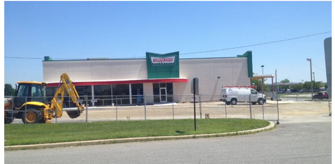
Crews finish up exterior work on the new store. (Doug Rainey photo)
