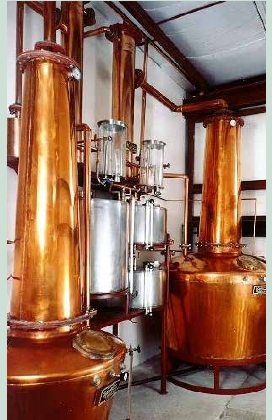
A Vendome system that will be installed at the Dogfish Head Milton site.
